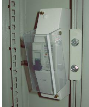
Circuit breaker (40Amp)
